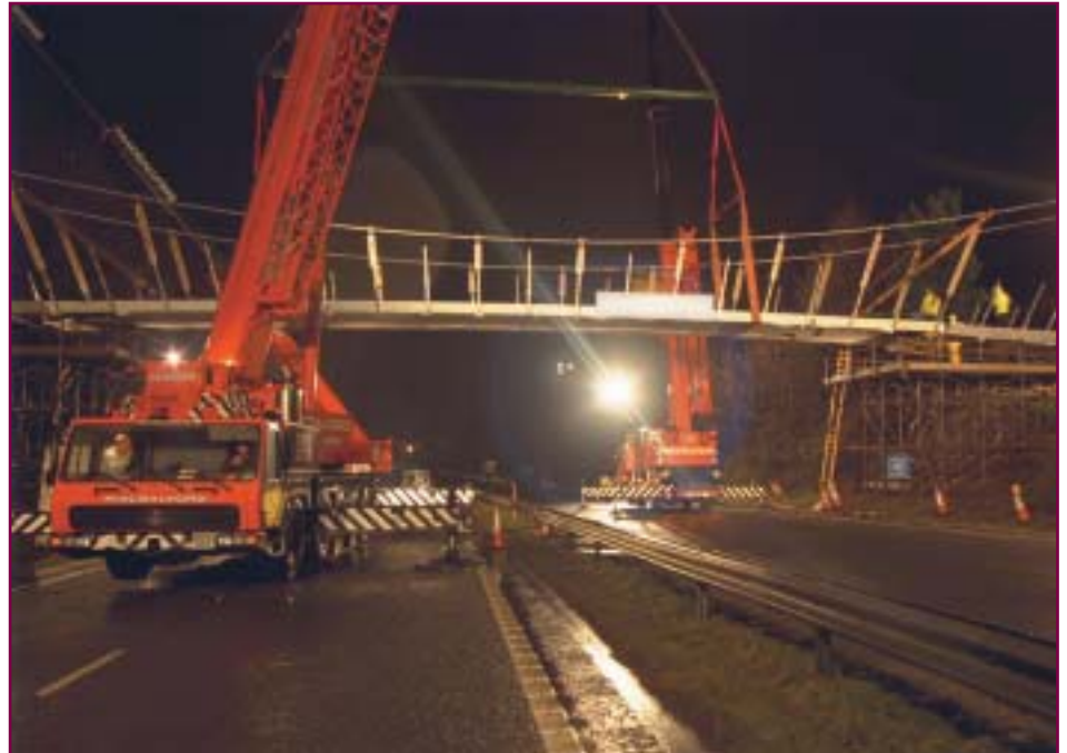
Overnight construction of the HA's first plastic footbridge over the A30. The HA will soon be constructing its first plastic road bridge.
