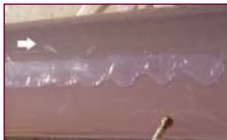
An air-pocket in a near-horizontal pipe
