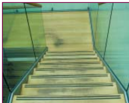
Uneven wear on timber stair treads and landings change slip resistance characteristics over time
