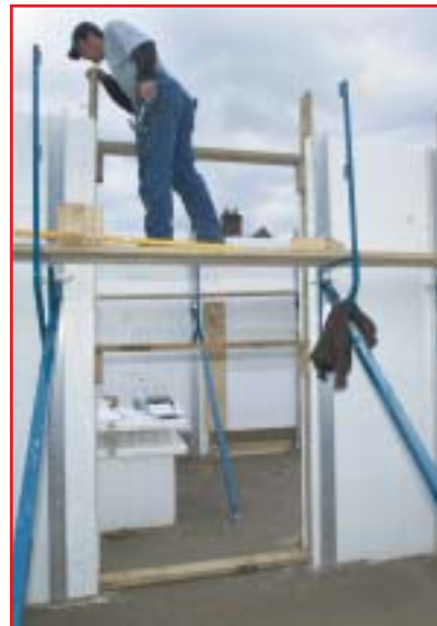
(Top) A Typical ICF Corner section (Above) A house being built using the ICF System
