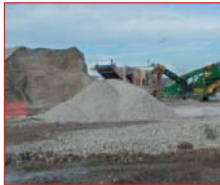
Crusting and stockpiling of crushed concrete from demolished paper-mill, at site of new regional distribution centre for Scottish & Newcastle Breweries, Thatcham (photo courtesy of Britpave)
