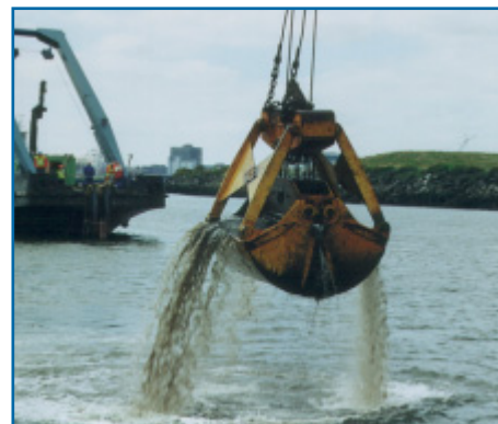
The grab appears to have fully closed but there is still significant release of material due to spillage from the top of the grab.
