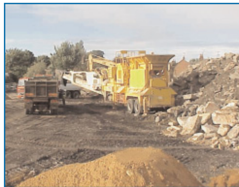
Effective re-use of materials such as concrete is a vital element of sustainable construction
