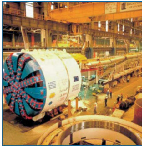
An Athens metro tunnelling machine – AGS-M is being used to help monitor geotechnical data.
