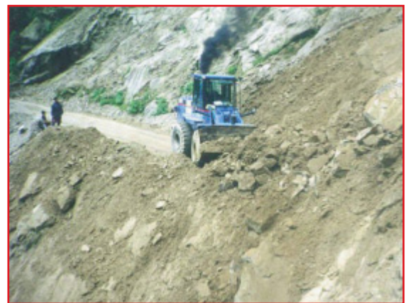
Landslides pose a major hazard to road maintenance in Bhutan
