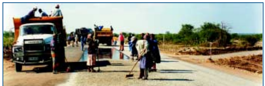
Surfacing a low volume road in Southern Africa using an Otta seal
